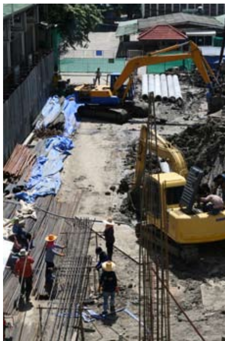
In the foreground workers are preparing the steel rods for the foundation
